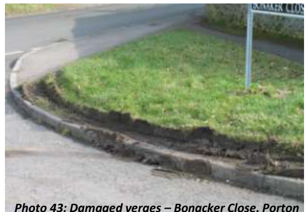
Photo 43: Damaged verges – Bonacker Close, Porton
